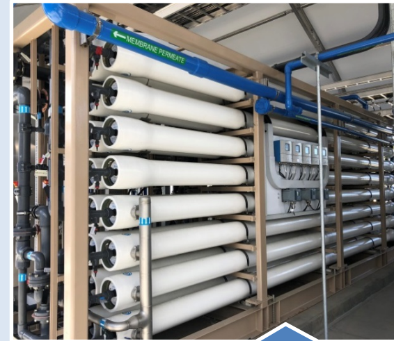
Future: Regional Recycled Water Program
